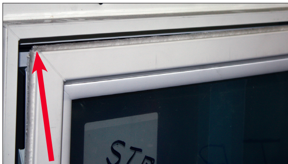
Window without Casement Corner Drive: Noticeable separation in the top corner of the window at DP75
